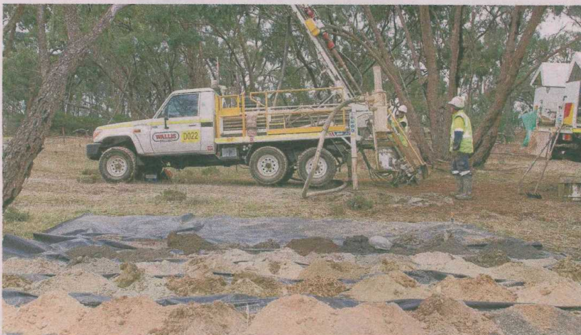
EXCITING: Works at the Irvine Gold Project near Great Western which uncovered more gold this week. PHOTO: Peter Pickering.
